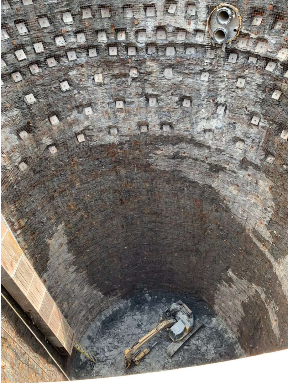
A view of the Enwave Well, under construction. (Enwave Energy) "It'll be 100 per cent heated and cooled by Enwave," said Carson Gemmill, the company's engineering lead for Toronto.
